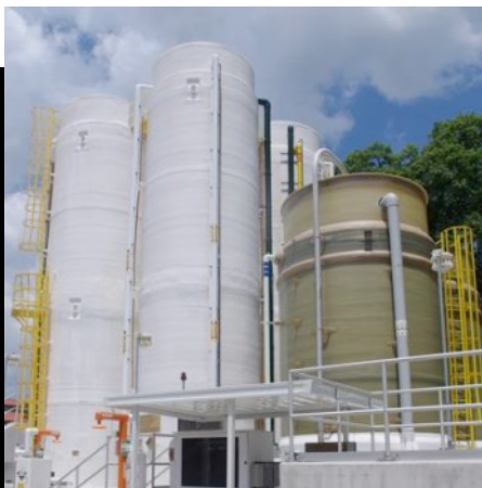
Omohundro Water Treatment Plant
