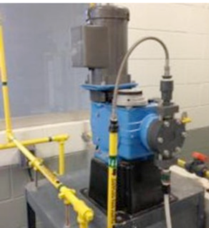
Encore® 700 Installation at Muttontown, NY
