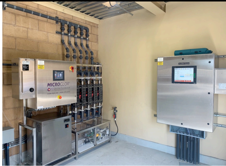
A Microclor® OSHG system installed at the Walnut Well in Santa Ana.
