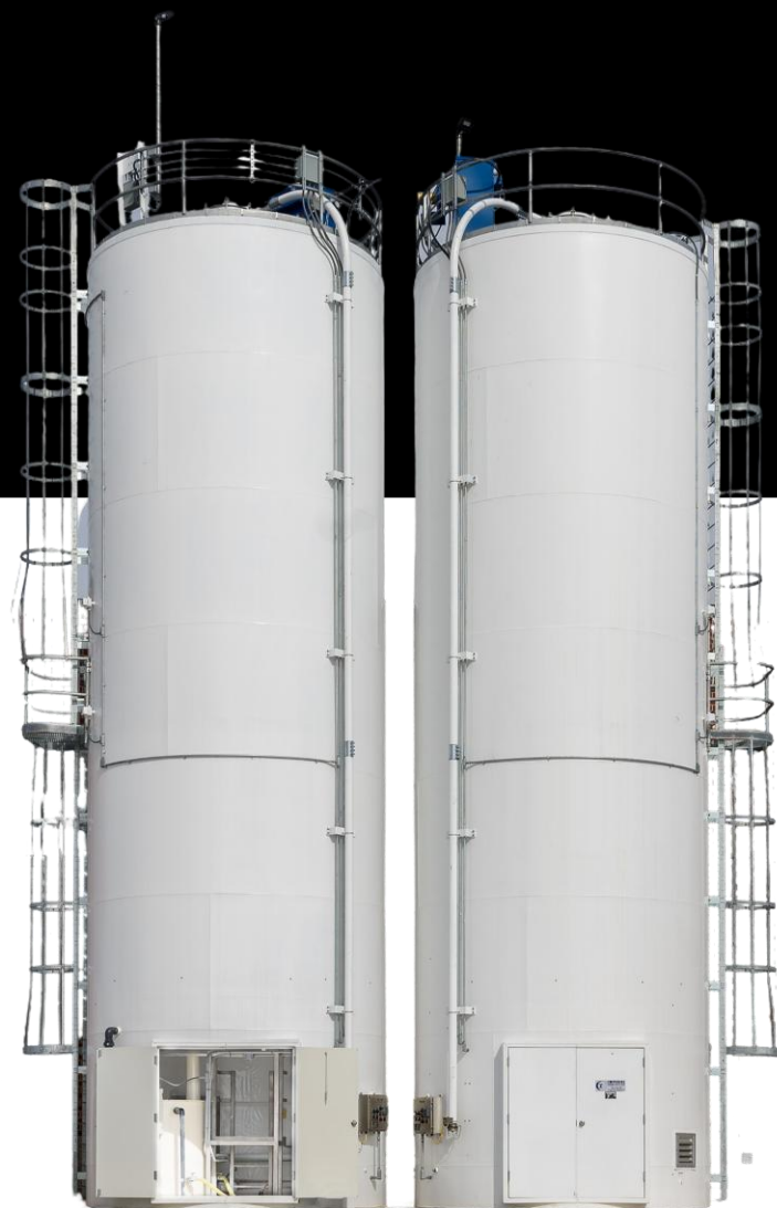
Bulk Chemical Storage and Feed System
