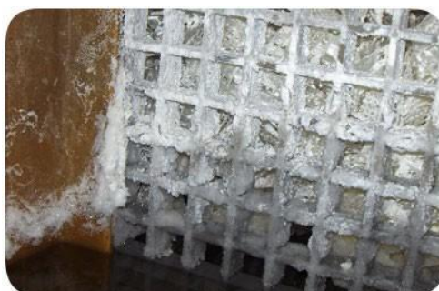
Packed Bed Before Acid Wash
