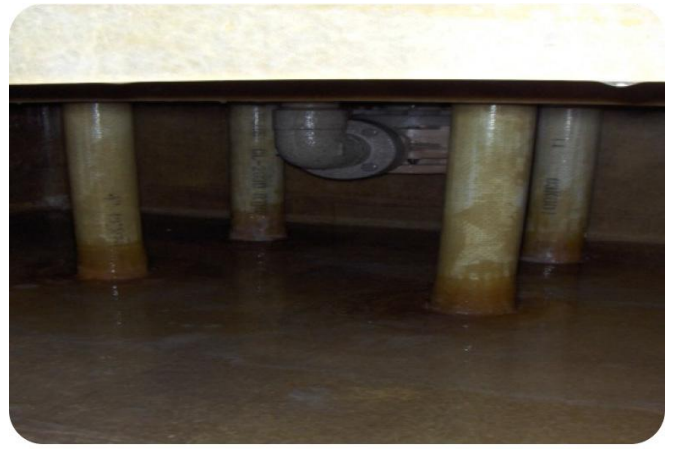
Sump After Acid Wash
