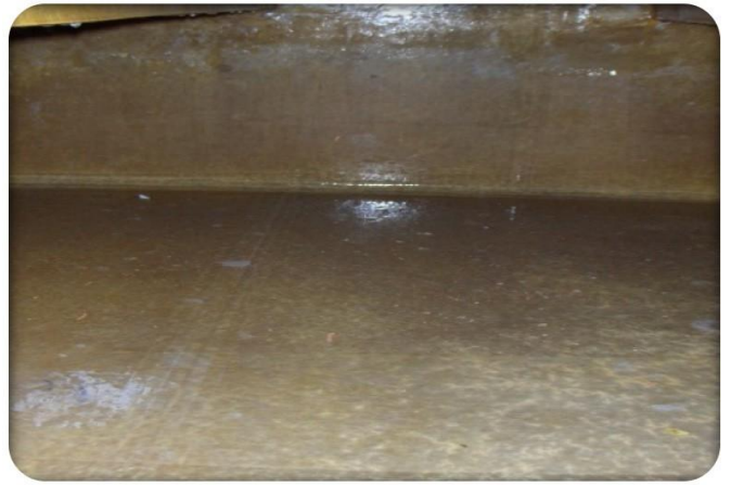
Sump after Acid Wash
