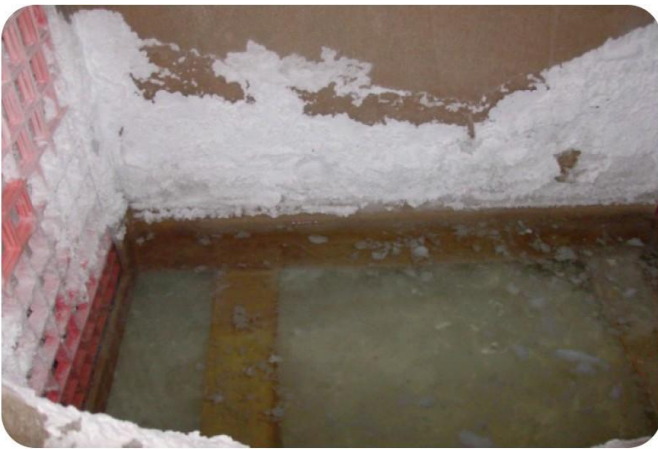
Solids in Sump Up to 29" Thick
