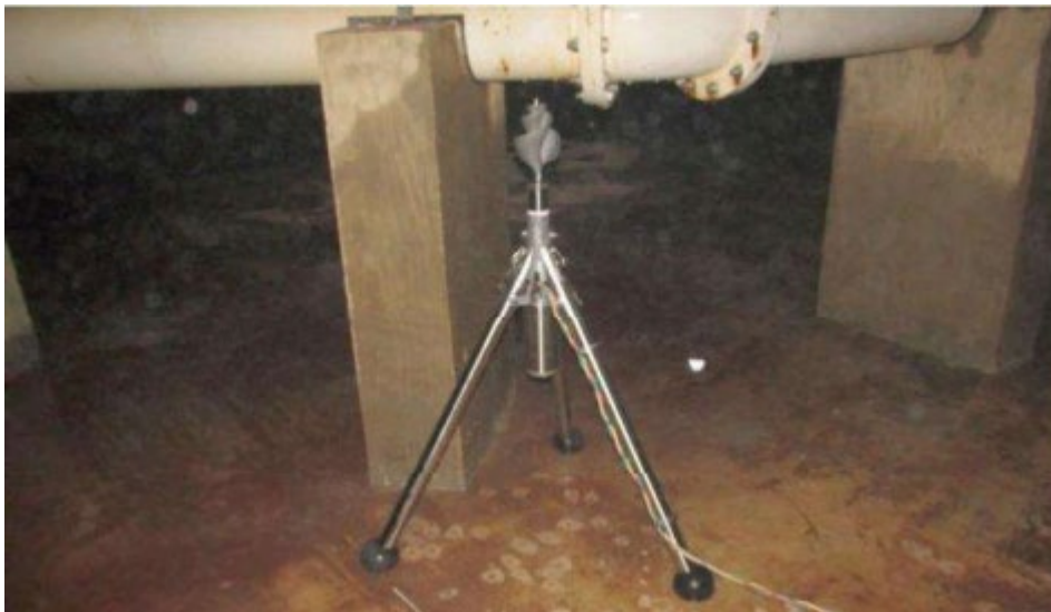
Figure 2. The PAX Mixer was installed in a 5MG tank with an existing passive mixer (shown behind PAX Mixer in above image).
