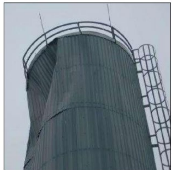
Winter ice formation can damage water tanks
