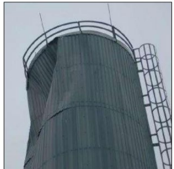
Winter ice formation can damage water tanks
