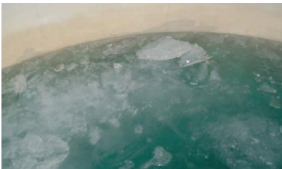
Figure 3a. Ice conditions inside the tank prior to turning on the mixer. Note the damaged coatings above the water line.
