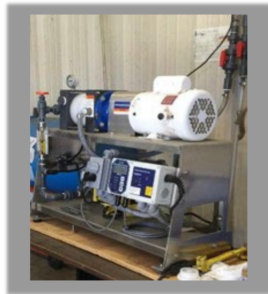
Polyblend® M-Series Pilot Unit at the Maple Creek WWTF
