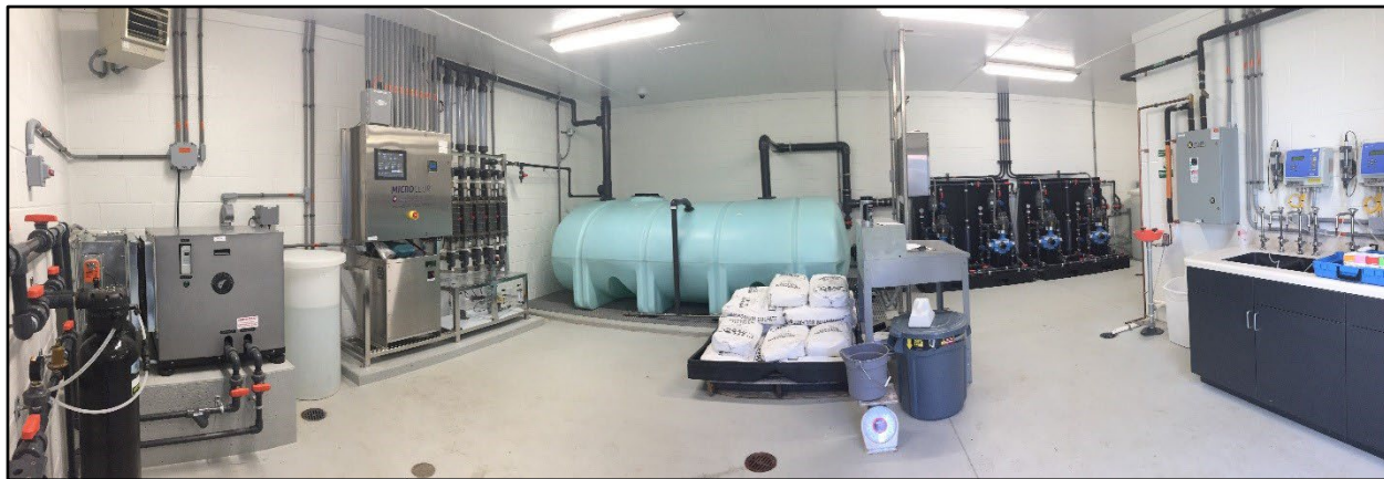
Figure 4 Monoclor® RCS residual control system with 100 pound-per-day Microclor® OSHG system
