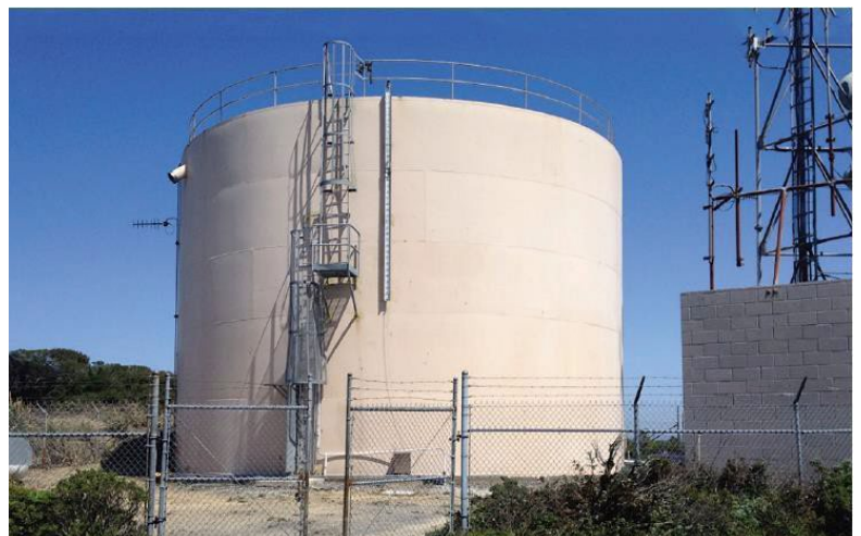
Figure 1. The 400,000-gallon Sweeney Ridge tank is the high point of the San Bruno Water system. While the tank enjoys some of the best views in the San Francisco Bay Area, the elevation, extreme weather and isolation by a 1-mile pipeline makes water quality maintenance a challenge.
