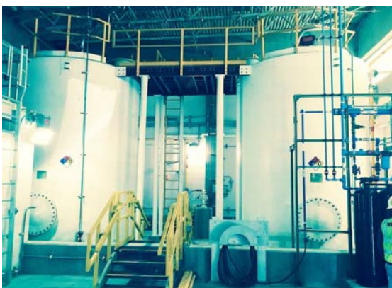
Hypochlorite (Bleach) Storage Tanks
