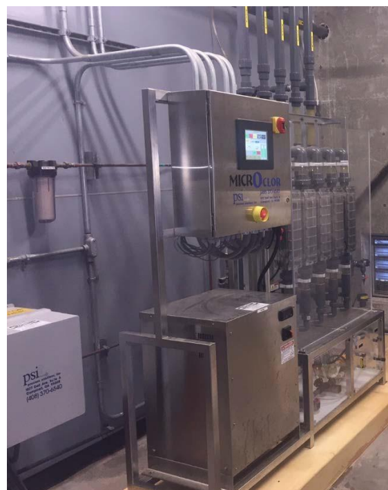
Nunes Treatment Plant 100 PPD Microclor® OSHG system
