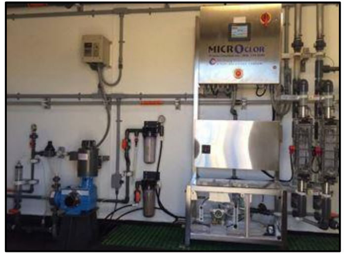
Inside the Monoclor® RCS trailer, the Microclor® OSHG
