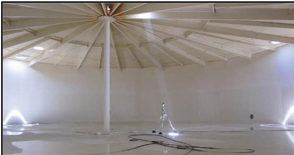
Figure 4. Interior conditions in the Ryan Ranch after cleanout and installation of the PAX mixer.
