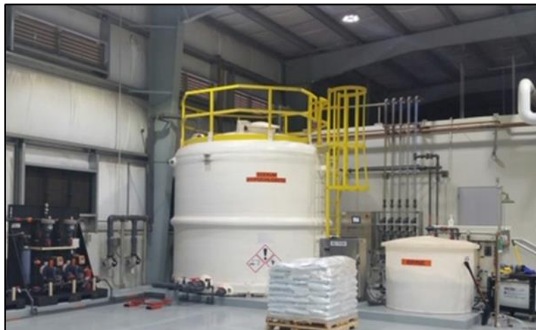
Hypochlorite storage tank, brine tank and pallet with bags of salt
