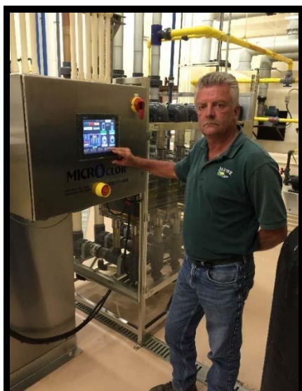
Kevin Cassady, Public Work Supervisor of Baxter, MN standing next to the 800 pound-per-day Microclor® OSHG system
