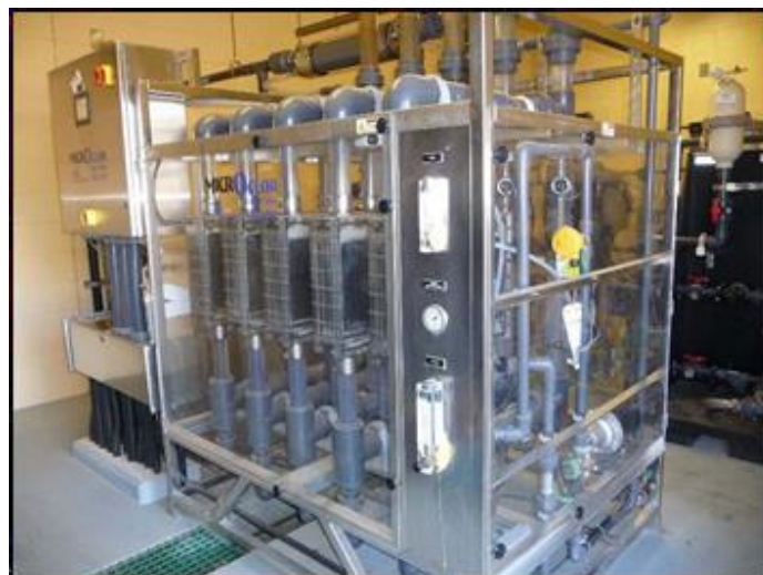
Wide angle view of softeners on the left, with one of the 800 PPD Microclor® OSHG units on the right
