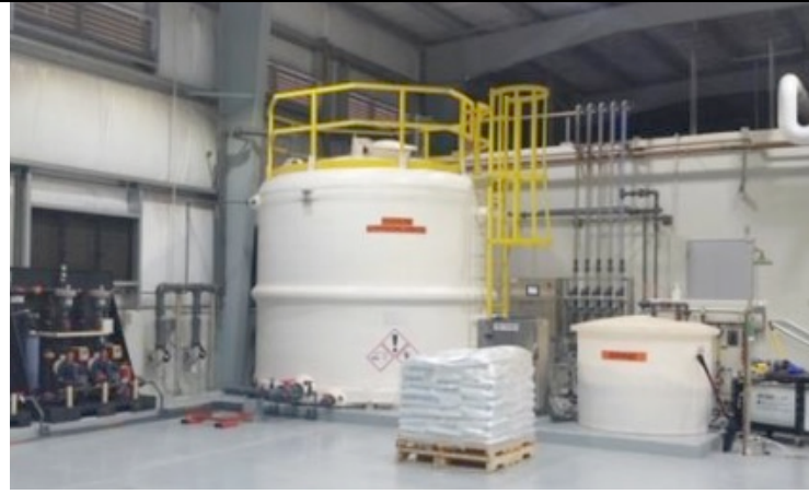
DSW Hypochlorite storage tank, brine tank and pallet with bags of salt.
